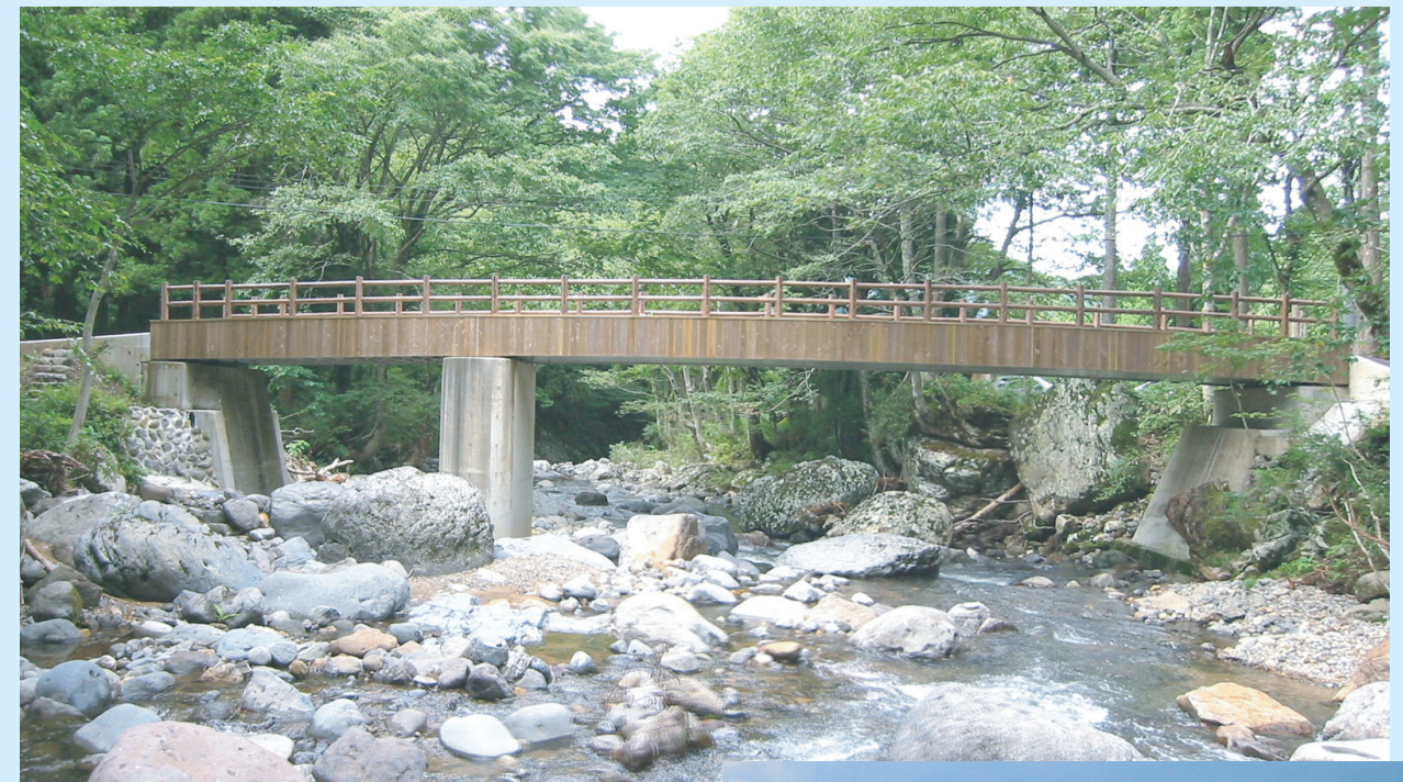
Works for changing the superstructure of Kubo Bridge, Bridge length: 24.80m (7.40 + 17.40) Komatsu City, Ishikawa Pref. (Built in May, 2004)
